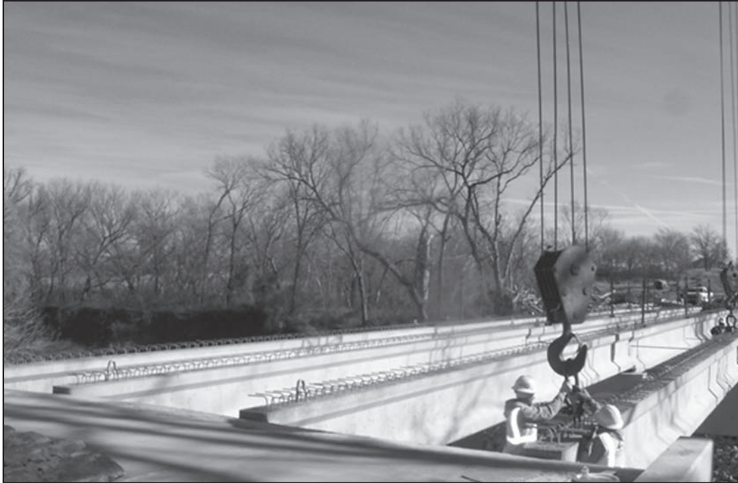
Cranes larger than the men who control them are used to lay the concrete beams. Picture taken Jan. 11, 2012.
