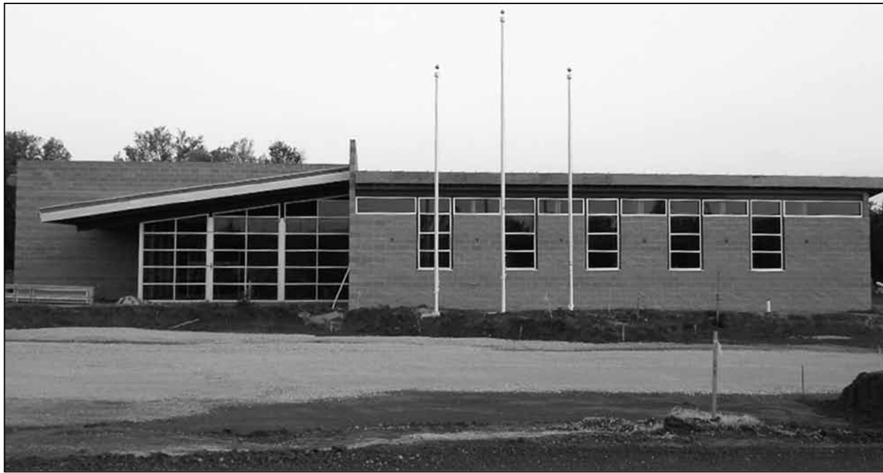
The Pawnee Nation Law Enforcement Center reaches the final stages in construction.
