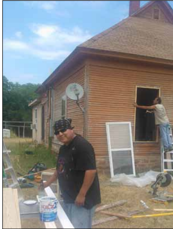
Dusty Eaves (front) prepares the new trim boards while Ronnie Cooper continues to reframe.
