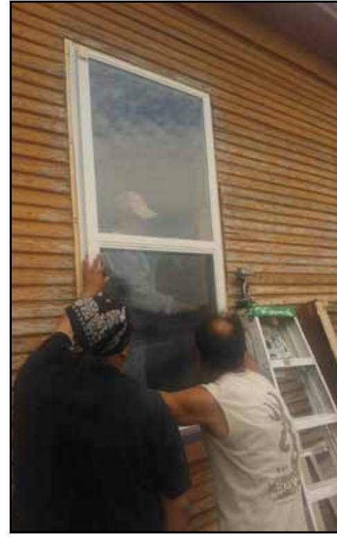
Dusty Eaves (left), Ronnie Cooper (right) and Sonny (Arthur) Fields (inside) install and seal the new, double-glass windows.
