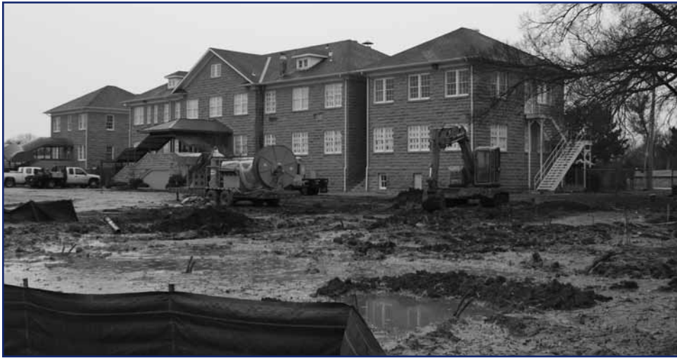
Ground Source Heat Pump being put into the Health and Community Center
